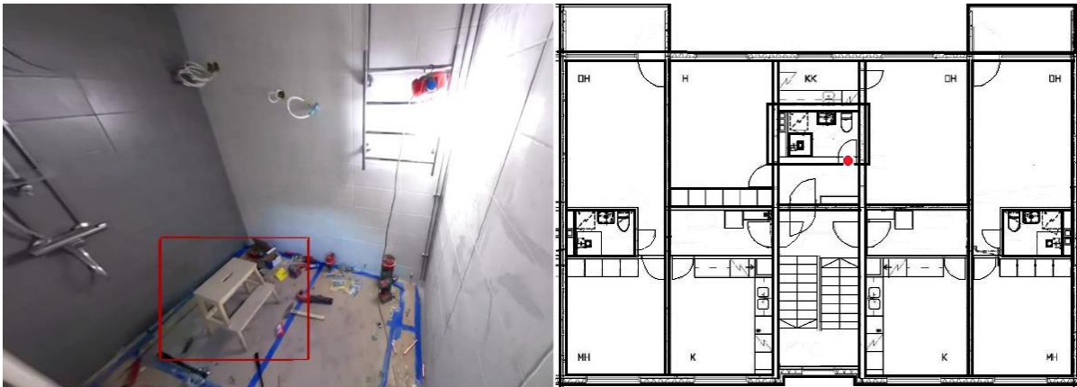
Fig.1. Left: A processed video frame with a red bounding box annotation pointing out that an unsafe ladder is used. Right: The red dot indicates the current location of the camera on the floor (plan) map.
