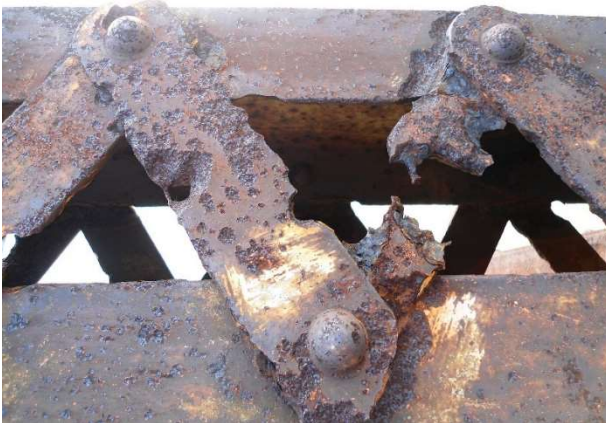
Image 1. Shows what a steel structure can look like when it has broken due to rust formation. (Wikipedia, 2023)
