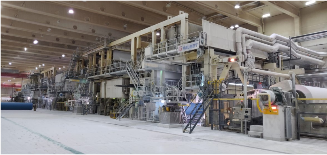
Picture 3. Coating machine (Strömberg, 2023)
