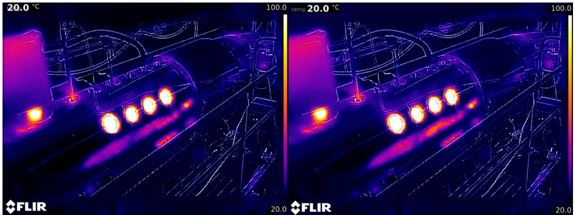
Figure 12. Temperatures 50 minutes after the exhaust gas pipeline had started heating up. No leakage on the left, artificial leakage on the right.
