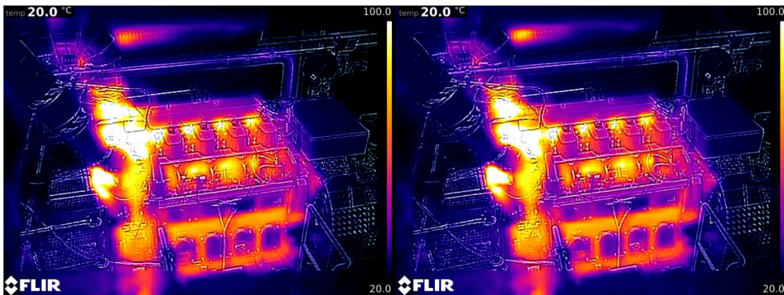
Figure 30. Temperatures at the load command to 100 %. No leakage on the left, artificial leakage on the right. Experiments on 3.3.2020 & 4.3.2020.
