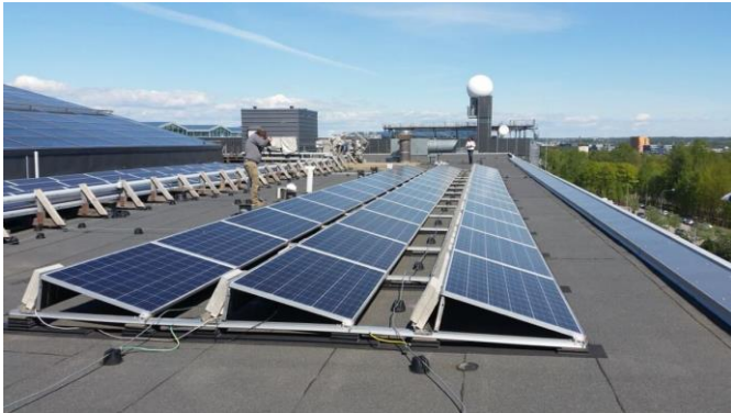
Figure 4.2 Installation PV on Helsinki Kumpula (Finnish Meteorological Institute, n.d.)
