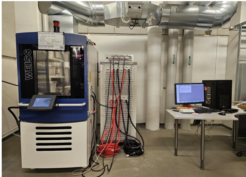
Figure 15. Battery testing facilities at VEBIC (WEISS thermal chamber, Neware BTS8000 and BTS4000 cycler and connector, data server)
