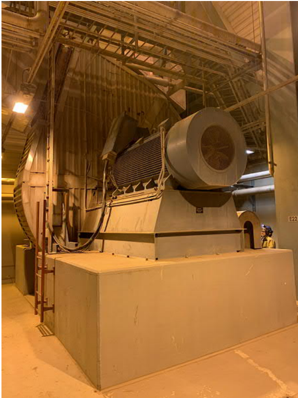
Figure 27 A fan powered by an induction motor, at Alholmens Kraft.
