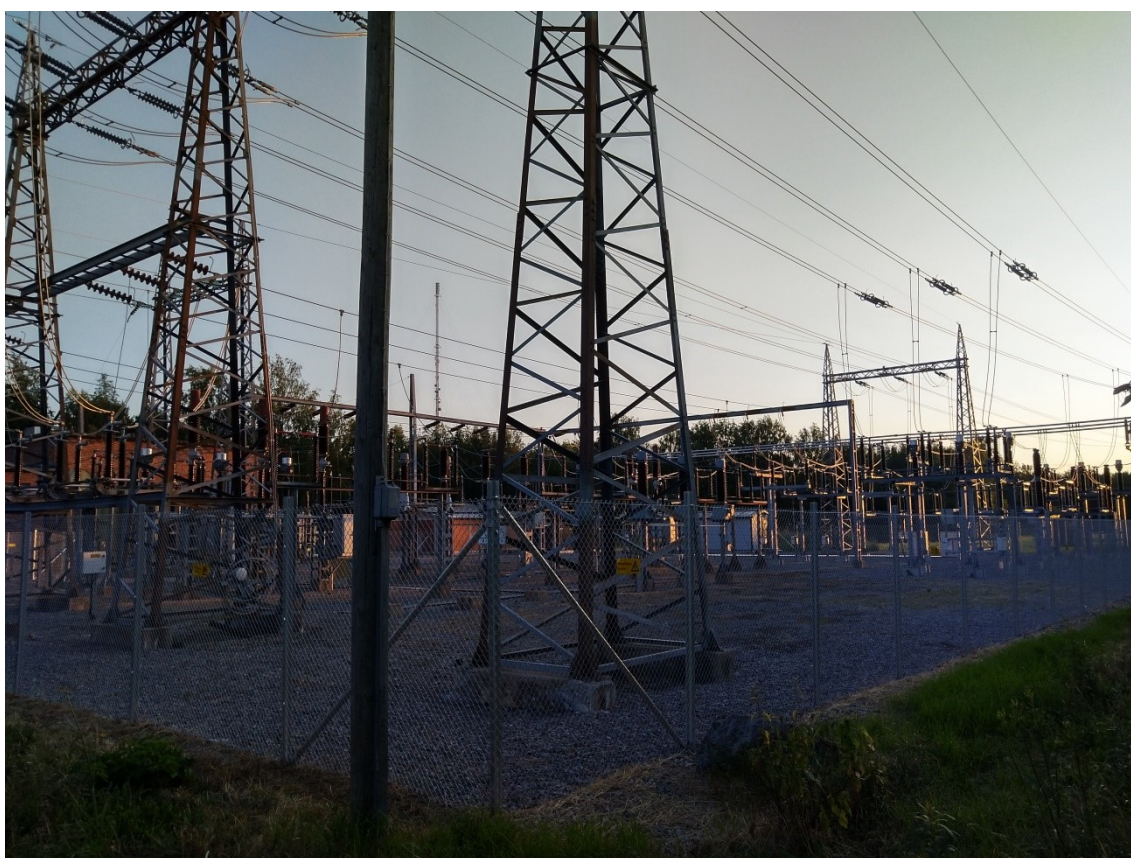
Figure 2. Purola substation area in Vaasa.
