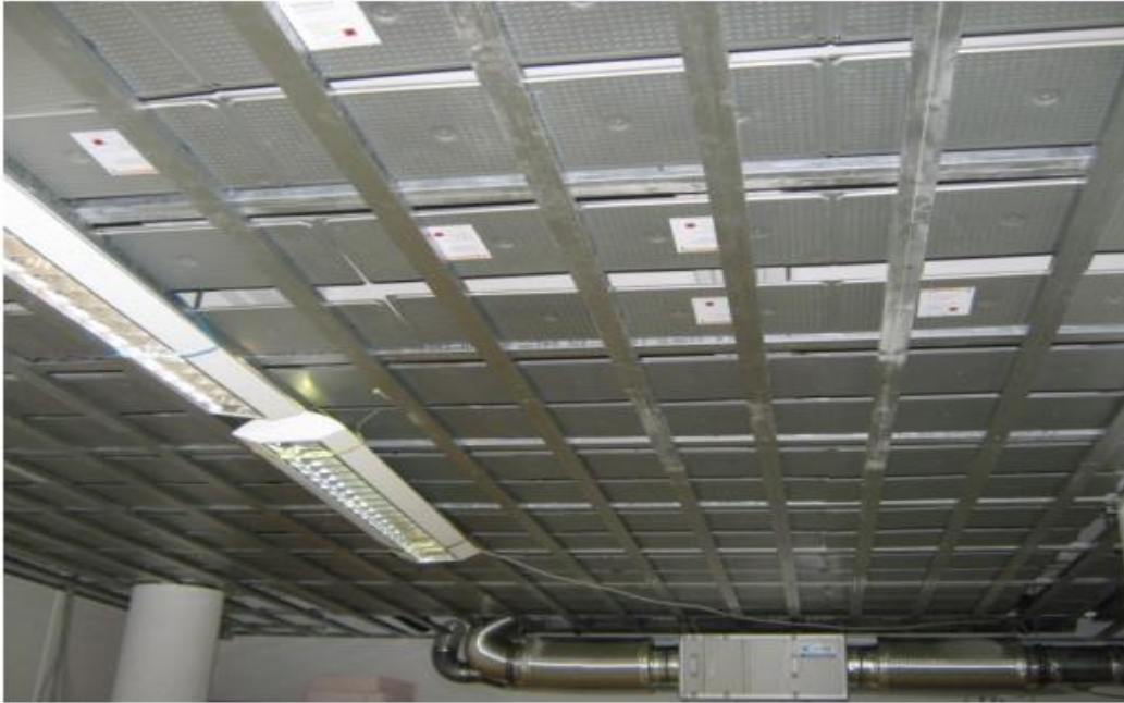
Figure 29. Installation of the phase changing material boards in the conference room ceiling (H. Weinlädera, W. Körnera and B. Strieder, 2014)
