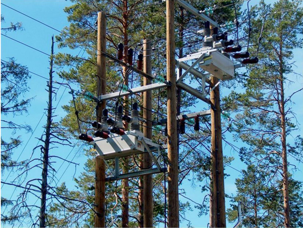
Figure 20. Sectionalisation of a rural network feeder with remote controlled line reclosers in the central regions of Finland.
