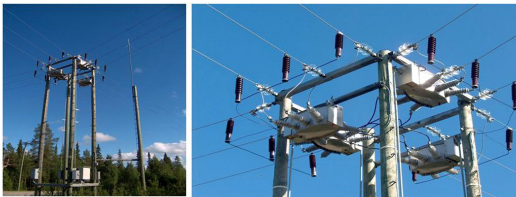
Figure 18. A distribution substation with SF6-insulated pole load-break switches in Lapland in Northern Finland.
