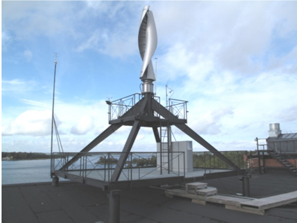
Figure 58. WS-4B wind turbine at field site at University of Vaasa, Finland.
