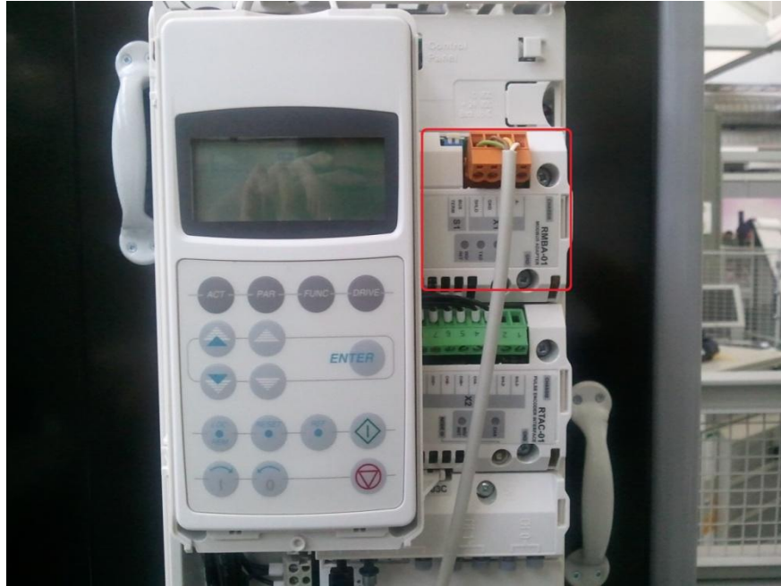
Figure 54. Modbus Adapter Module installed on ACS800's control panel (area marked in red rectangular).
