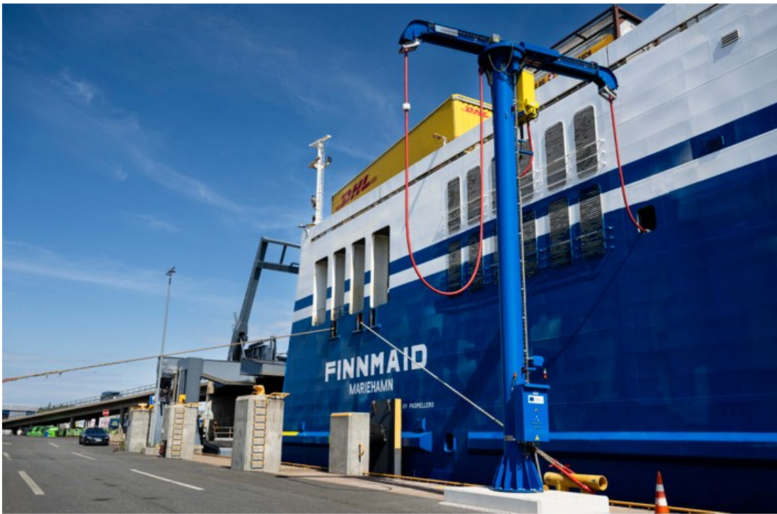
Figure 5 M/S Finnmaid is attached to the onshore power supply system in Quay C at Vuosaari Harbour. (Port of Helsinki, 2024)
