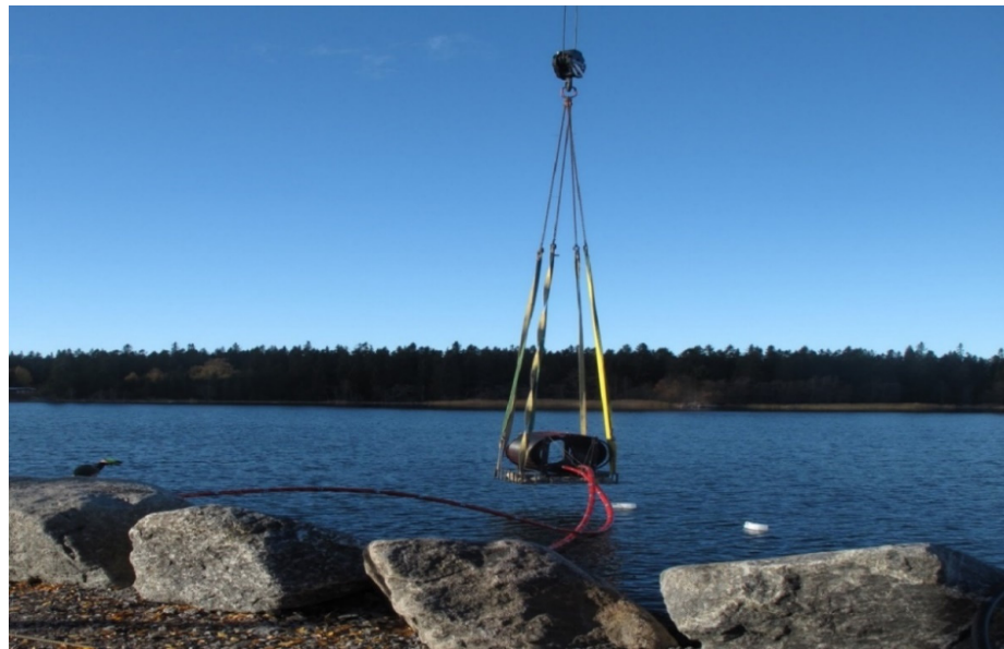
Figure 4. The water heat exchanger being put inside the sea shore at Merten Talo (Picture taken by Anne Mäkiranta during installation process 18 October 2018).
