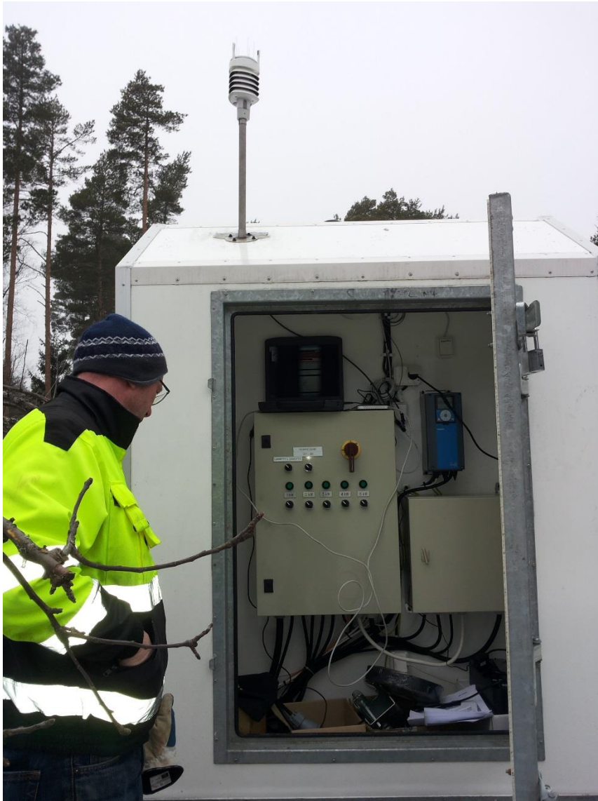
Picture 9. Weather tower and measuring closet.
