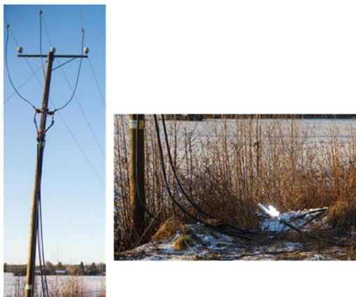
FIGURE 9. Earth fault field tests (photo credit: Jukka Rinta-Luoma).
