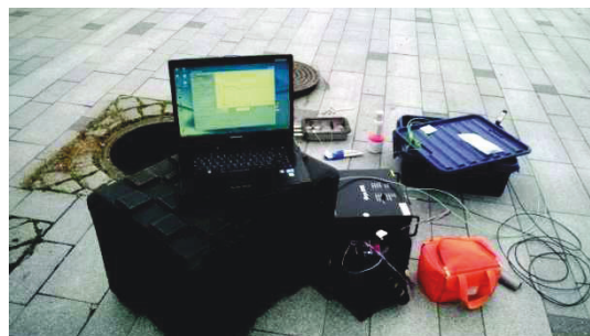
Figure 1. DTS-device was in commission at the low energy network site in Suvilahti.
