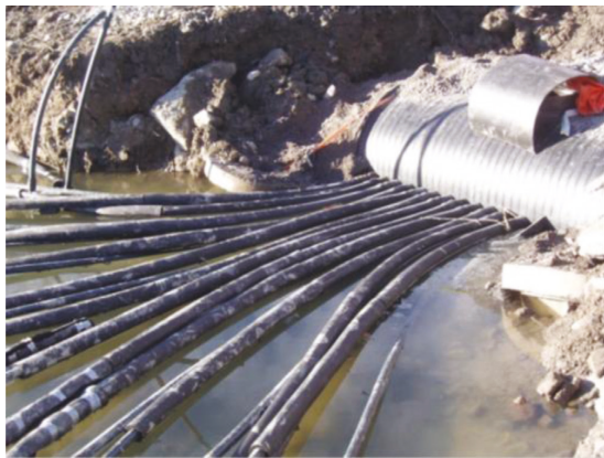
Fig. 5. A heat collection well performed as a link between heat collection pipes and the distribution well system. The image shows the actual connections between pipes and well installed in Suвилаhti.
