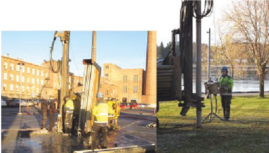
Figure 4. Drilling of measurement wells in the parking lot and lawn field was done in the late Autumn 2013.
