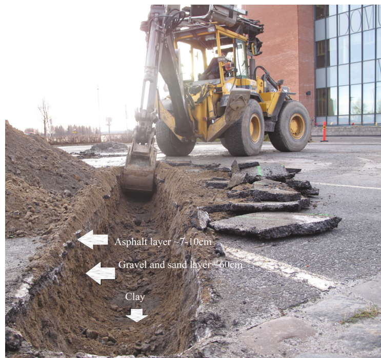
Figure 5. Soil layers under the asphalt in the measurement field at the University of Vaasa campus area.
