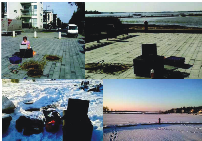
Figure 1. The measurement site is located in Ketunkatu street. A box including optical fibers with connectors is placed in the distribution well.
